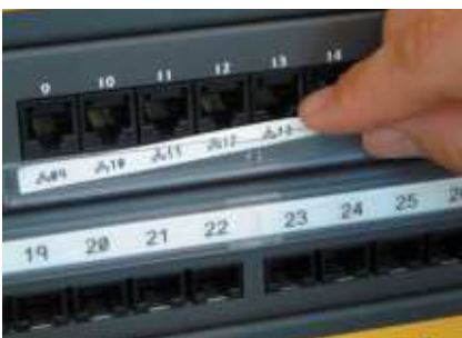
Punch block & patch panel labels
